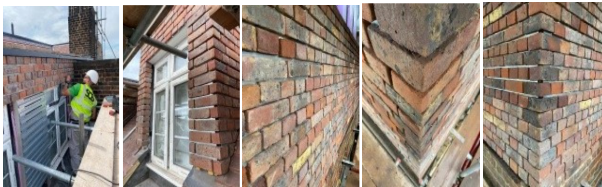
Cedar Hall School London, We Built Up two floors with steel then Fixed our system to an SFS
