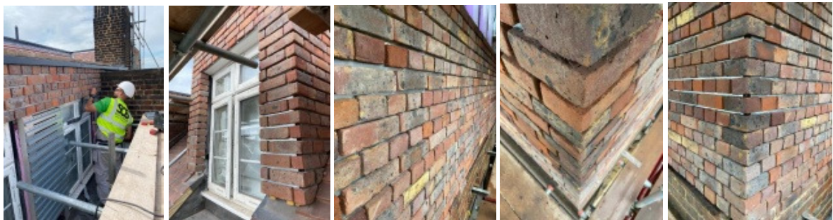
Cedar Hall School London, We Built Up two floors with steel then Fixed our system to an SFS
